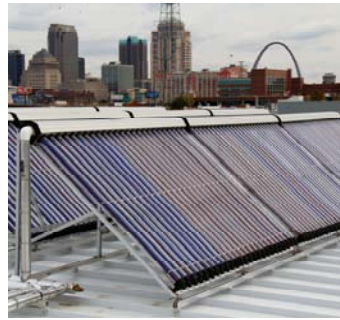
Solar thermal on the roof of the Sheet Metal Workers' Local 36 new headquarters
